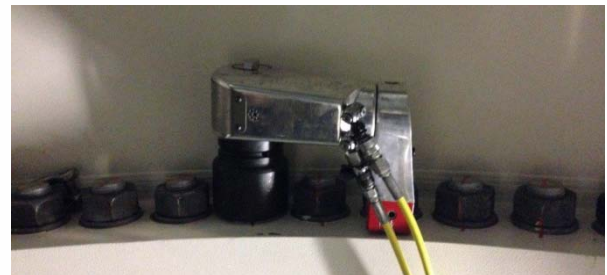
Figure 5: alkitronic® Hydraulic torque wrench AS-15 on tower flange bolts M64- high tension
